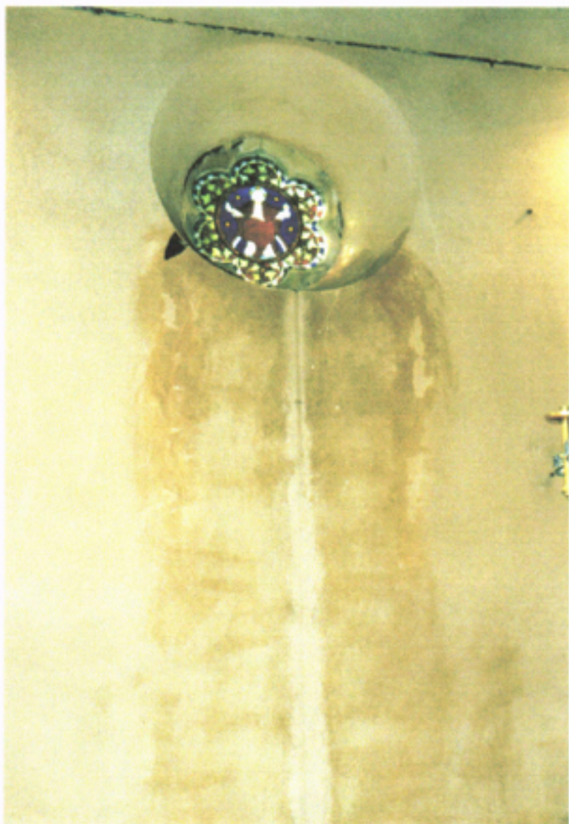
West wall rose window showing effect of water penetration on plasterwork
